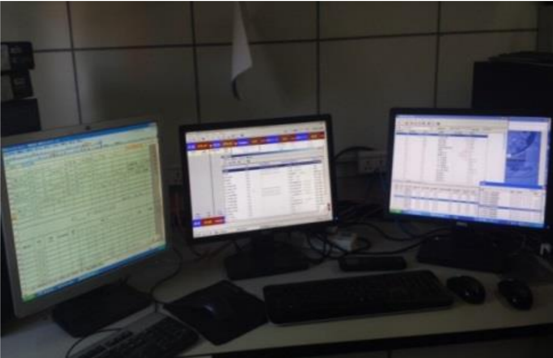
Monitoring indicator display terminal
